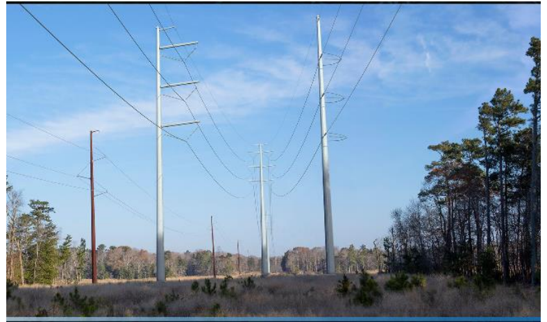
This photo rendering shows what the new galvanized steel poles are expected to look like along the rebuilt transmission line in Sussex County.
