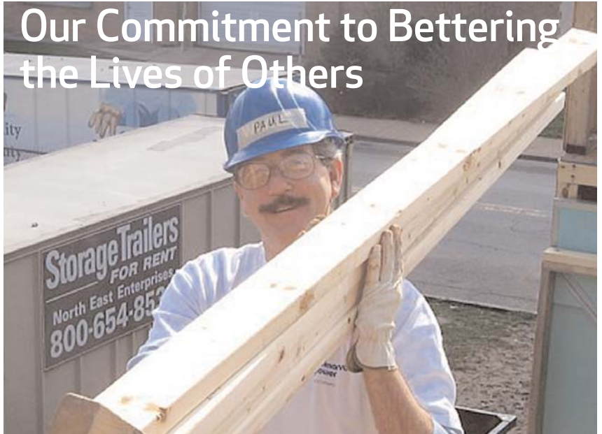
Paul Keffer, a Delmarva Power contract employee, helps Habitat for Humanity build a home as part of the Hope Landing revitalization project in Wilmington.
